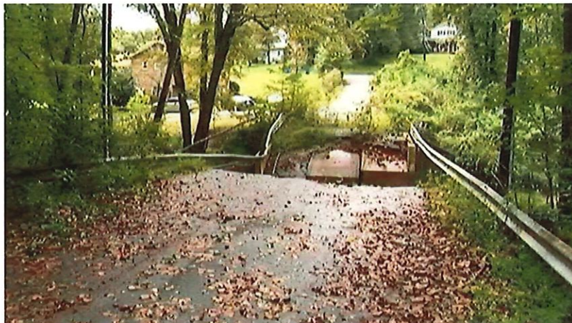
Photograph of the subject bridge taken after the incident in daylight
